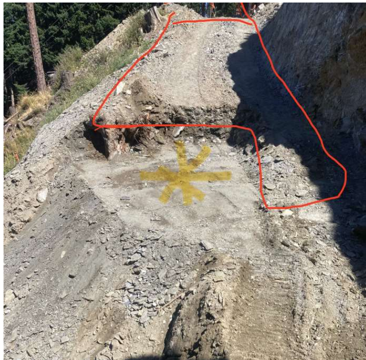
Photograph 2:- Site won fill (crushed rock) on southern ramp benched into slope (yellow *), Road lowered to remove fill material- Red outlined
