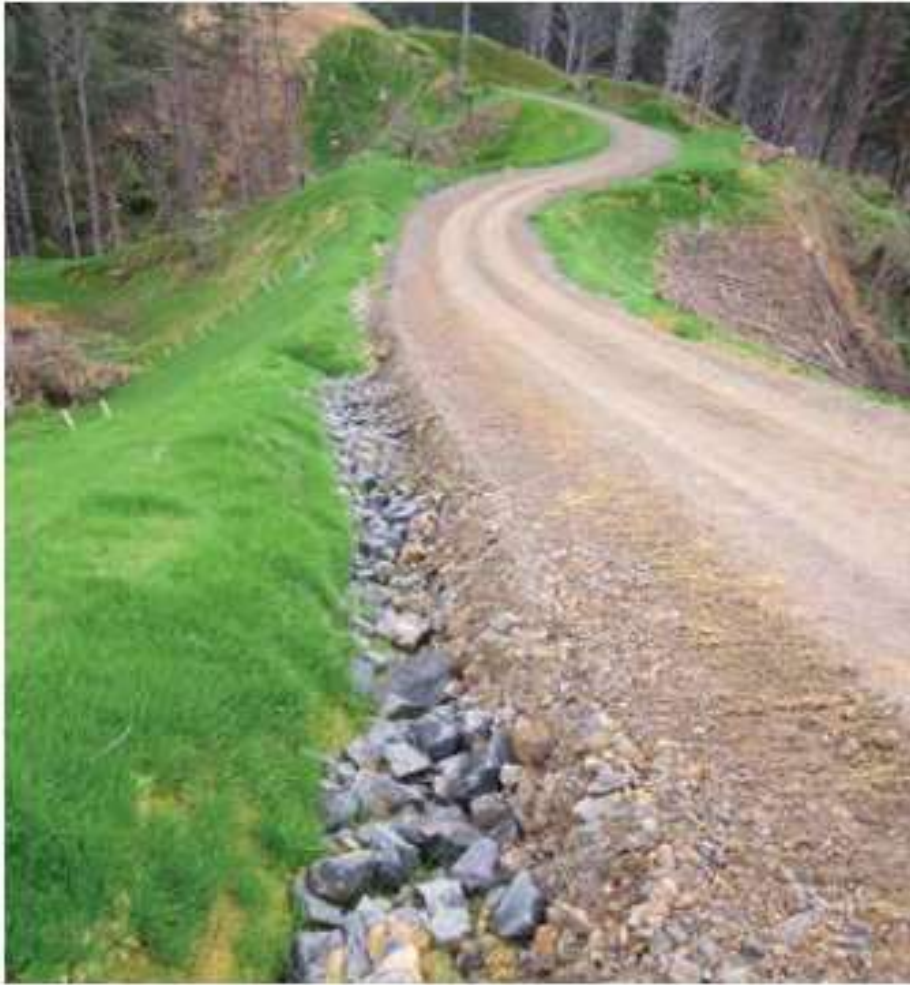
Photograph 5:- Suggested rip-rap lining configuration of a water table drainage ditch, as per NZFREM
