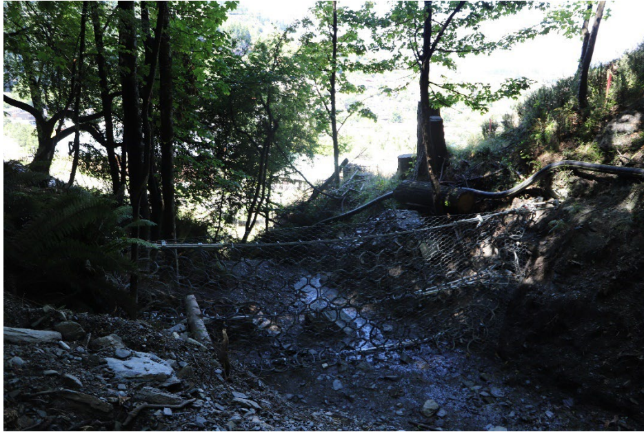
Photograph 1: Example of an existing debris flow barrier in the lower Reavers Creek catchment.
