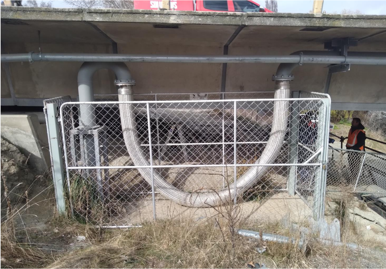
Figure 5-3: Existing Rockgas Gas Pipeline Configuration at Cromwell Abutment of Shotover River Bridge
