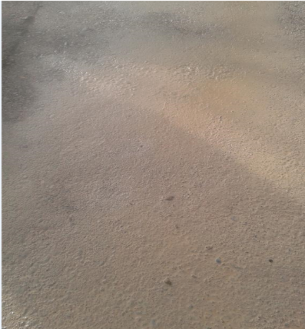
Figure 3 Aggregate wetted down during compaction to achieve 98% of MDD – note no compaction depression lines
