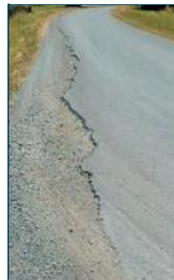
Figure 79: Sealed Pavement - Edge Break
