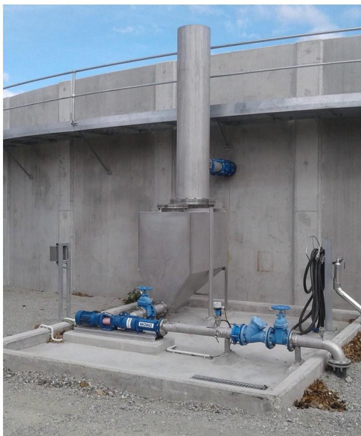
Figure 13 : Scum Pump Station
