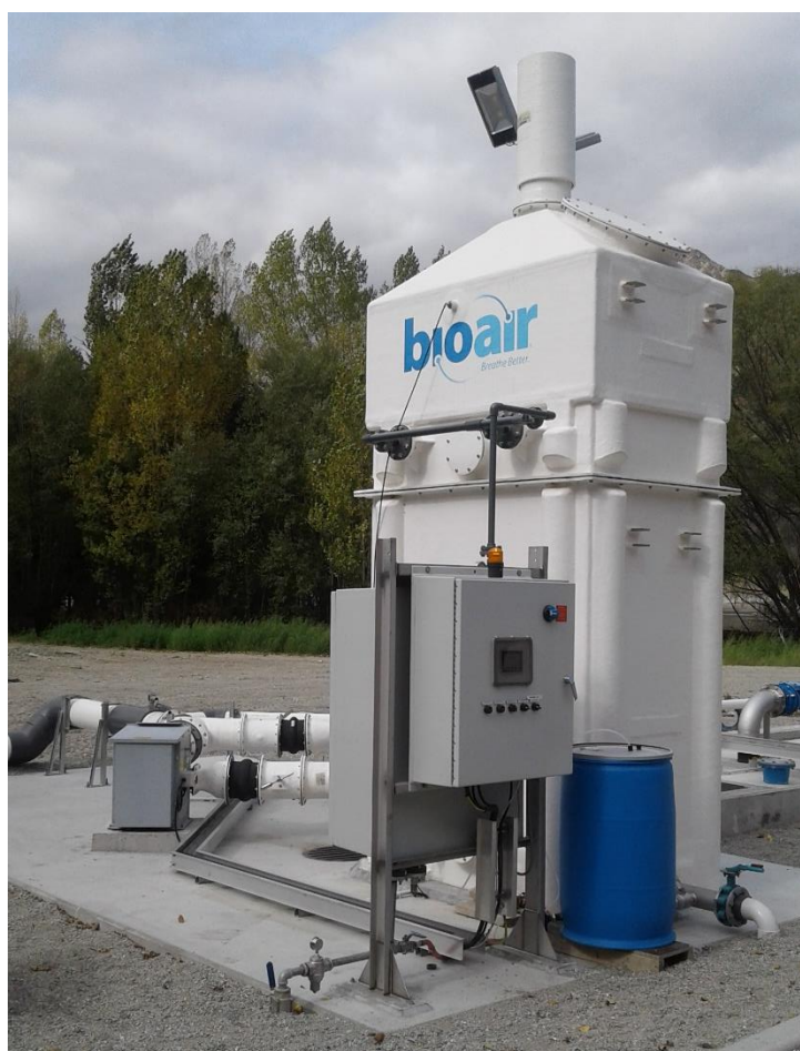
Figure 20 : Odour treatment plant
