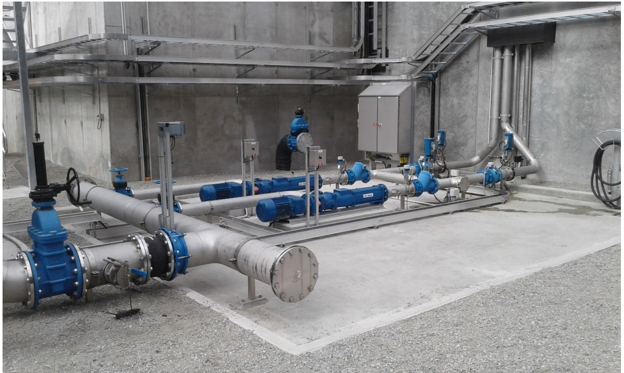
Figure 16 : WAS Pump Station
