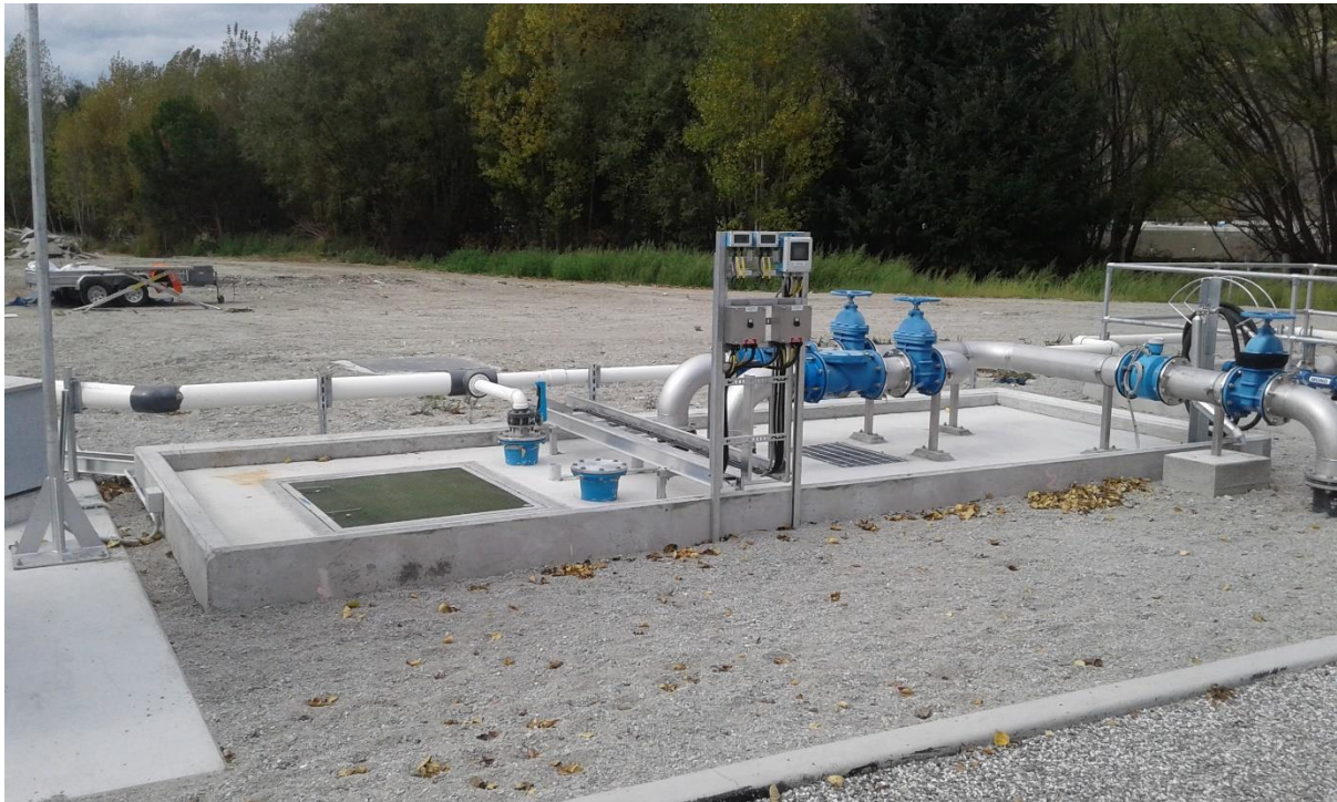
Figure 18 : Site Wastewater Pump Station
