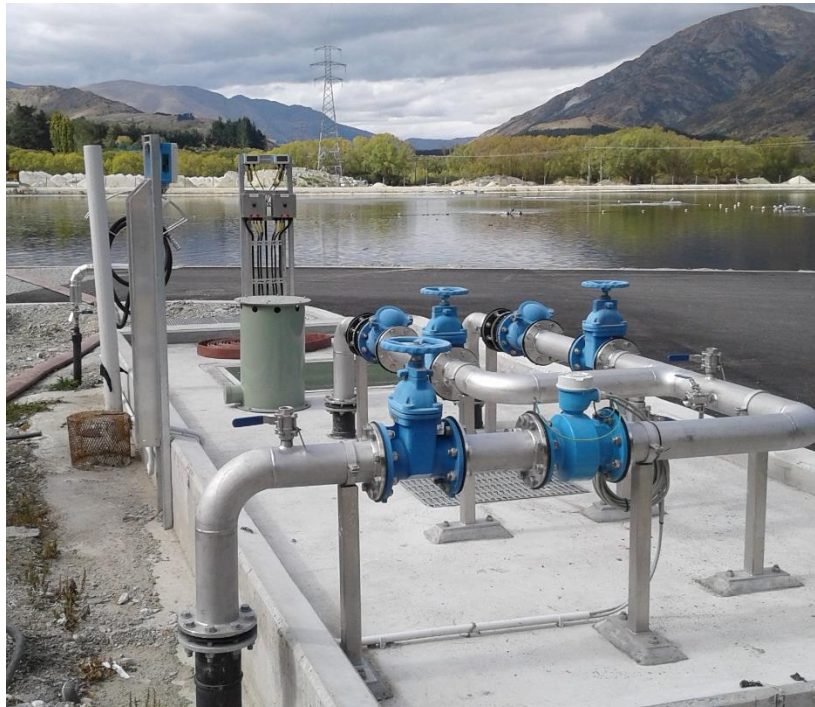
Figure 7 : Inlet Works Pump Station
