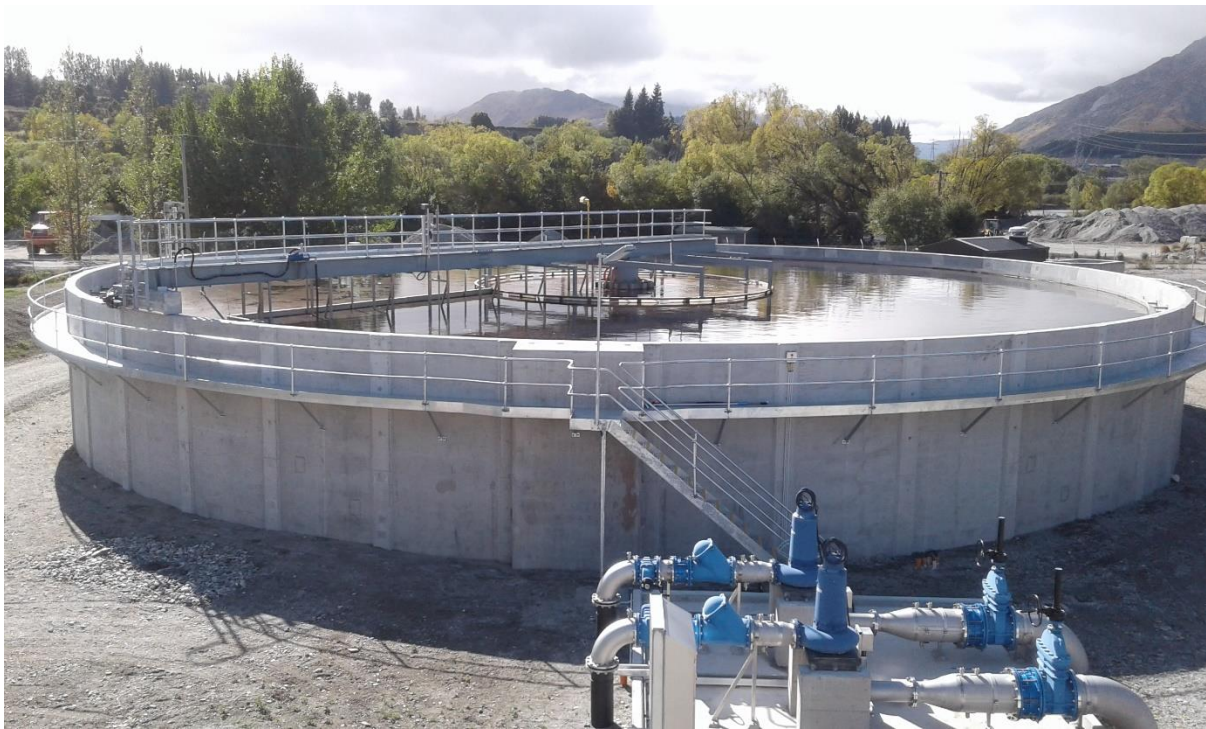
Figure 12 : Clarifier tank with RAS pump station in the foreground
