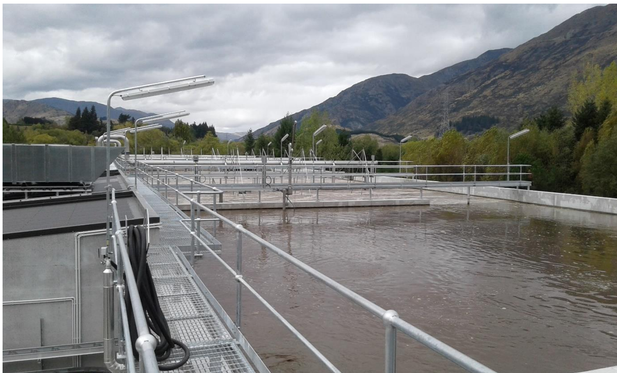
Figure 10: View across MLE reactor tank, viewed from anoxic zones
