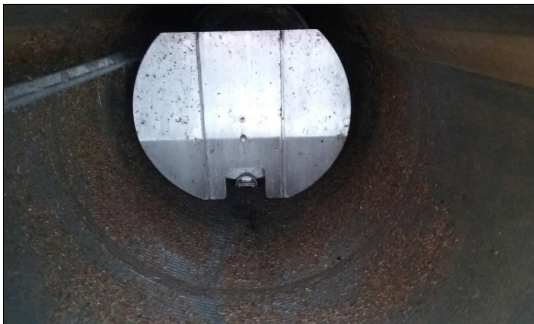
Figure 5 : Inside one of the drum screens
