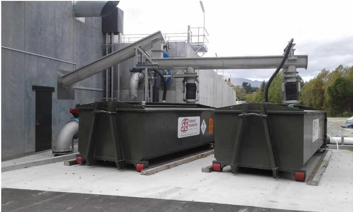
Figure 17 : Sludge conveyors and bins
