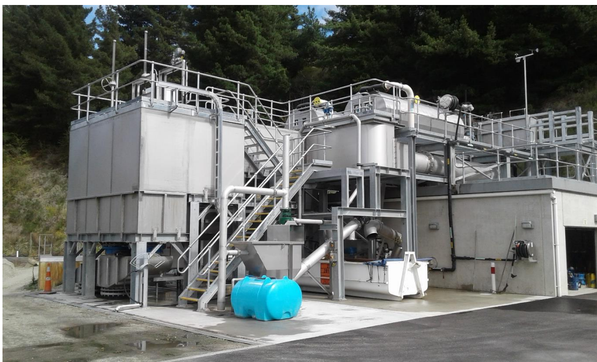
Figure 3 : Treatment Plant Inlet Works
