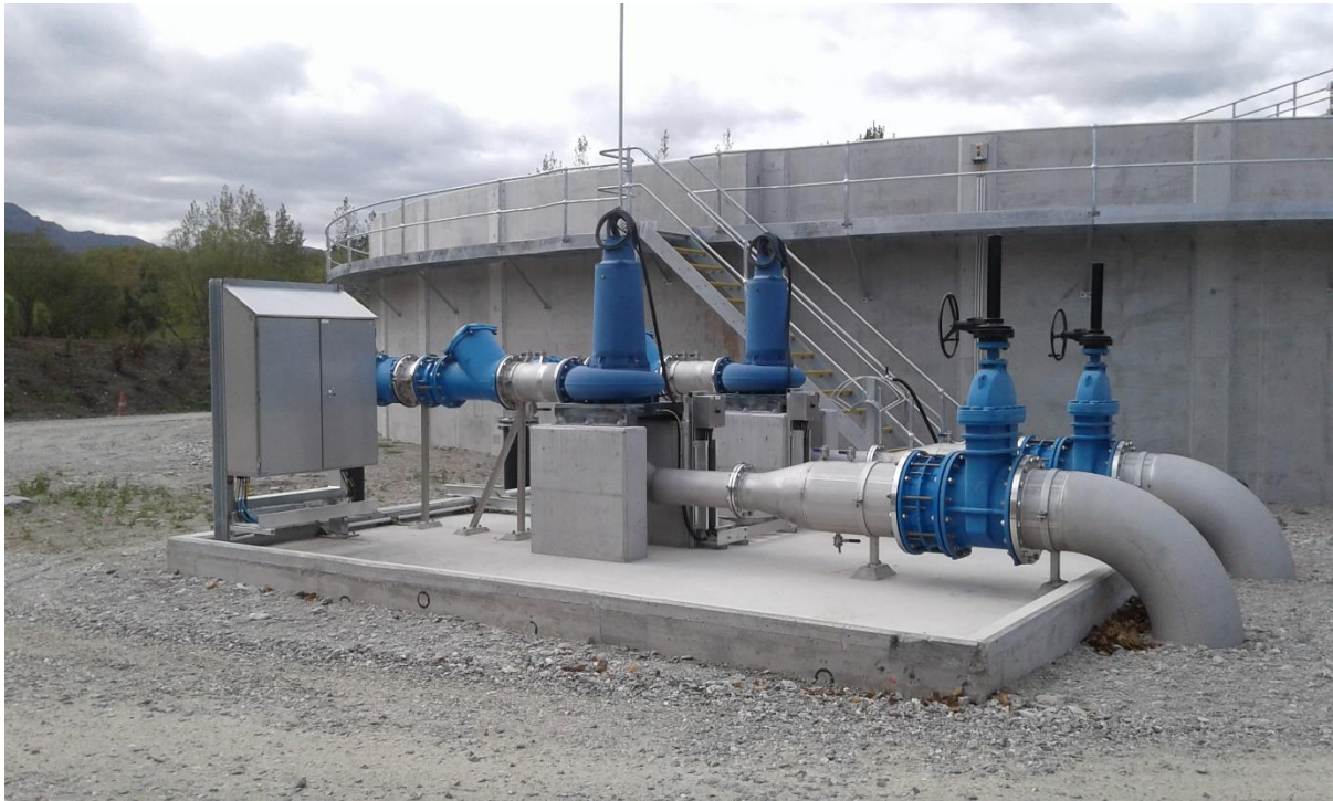
Figure 14 : RAS Pump Station
