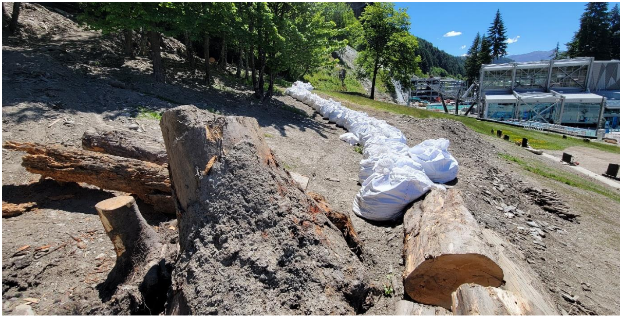
A temporary barrier was put in place to protect the recently cleared areas (above)
