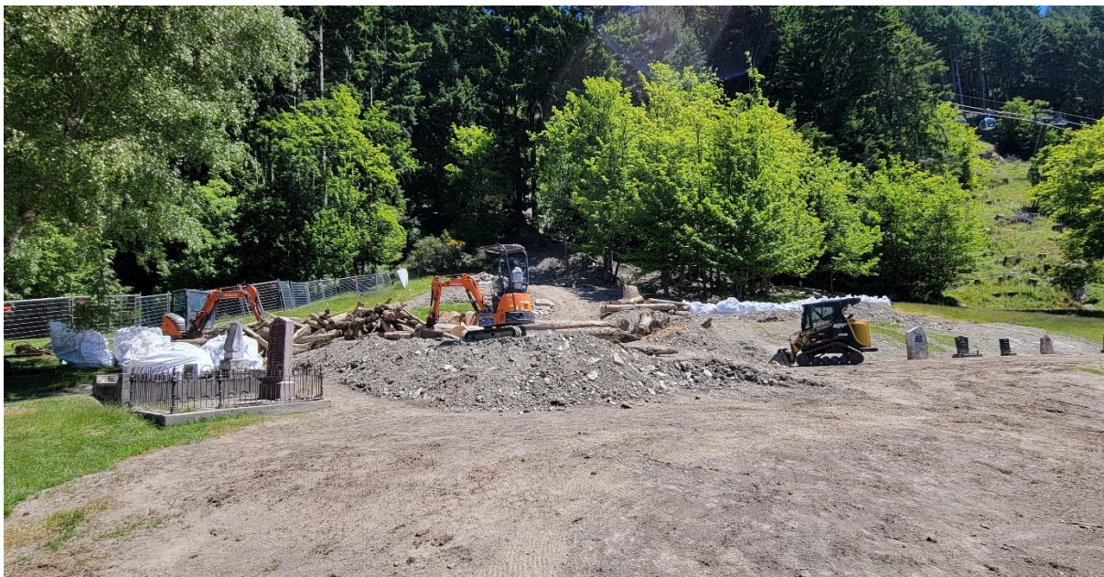
Works have now moved to the upper area of the cemetery (above)
