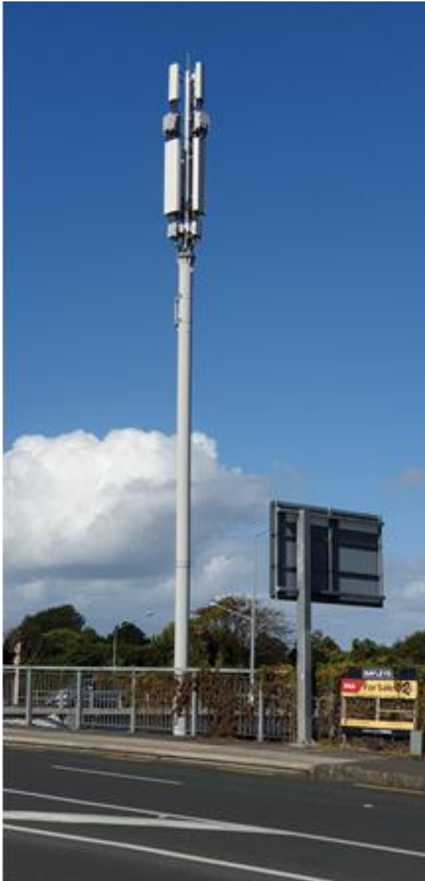
Figure 3: Vodafone facility with 'double cluster', Market Road Interchange Auckland Southern Motorway (example is 23m high). Indicative of a multiple operator scenario using cluster mounts.
