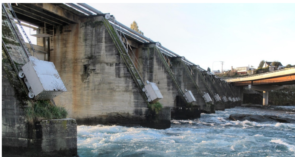
Fig 2. Gate counterweights which are likely to derail in a sufficiently large earthquake
