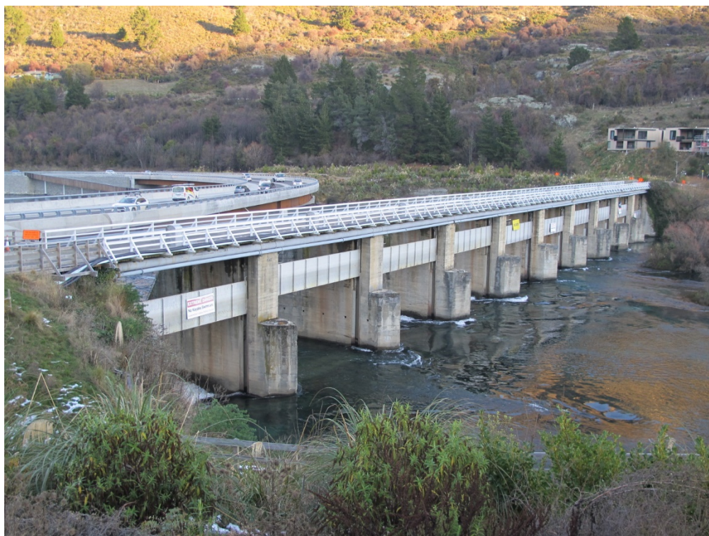
Fig 3. The gates in slots in the piers. Note water and power services above the gates
