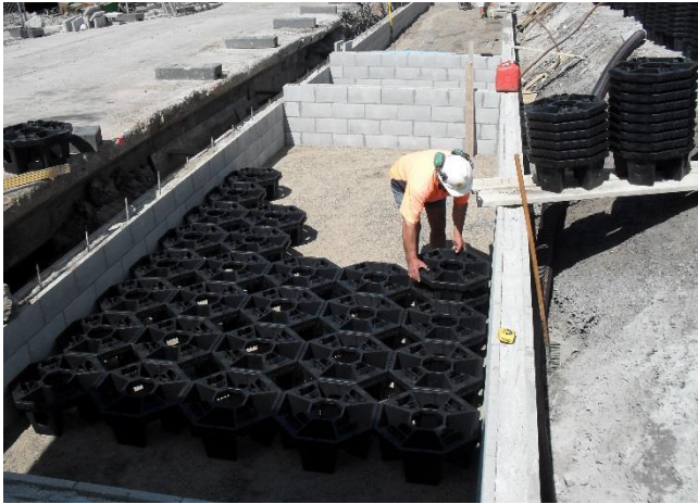
Integration of trees and infrastructure. Example of soil cells being laid out into tree pit areas. Image courtesy of Paul Malcolm, MetroGreen.
