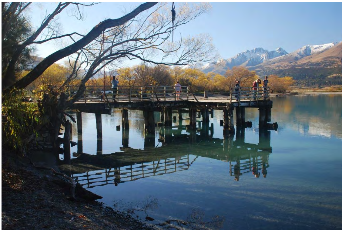
The southside of the jetty today – the end furthest from the shore is T-shaped. Truncated piles can be seen rising through the surface of the lake as the water level is low.
