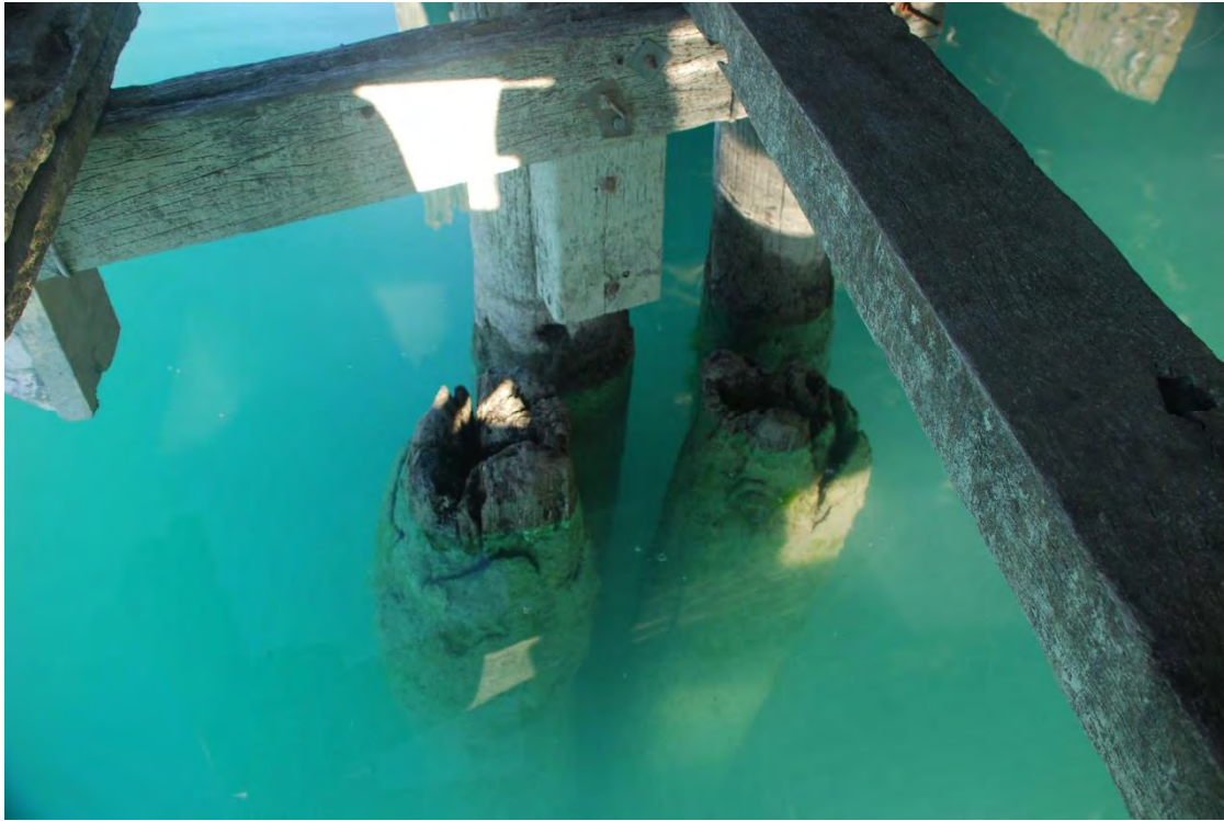
The remains of doubled-up piles probably dating to the first jetty of c.1873.
