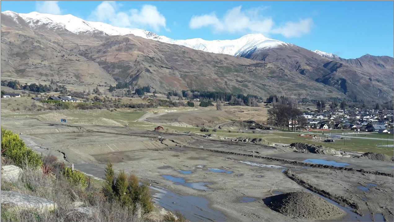
Figure 6: Open earthworks areas with no clear staging or progressive stabilisation
