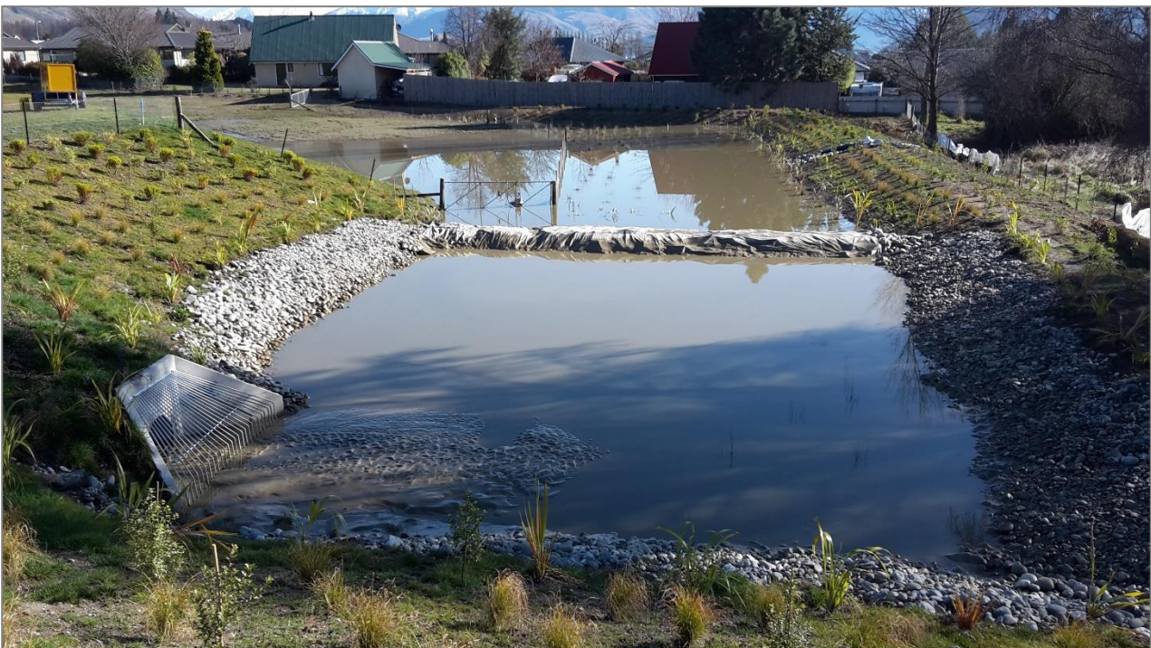
Figure 7: Sediment collected in a completed stormwater pond from Figure 6 catchment (the stormwater pipe was half full of sediment and will require extensive mucking out)
