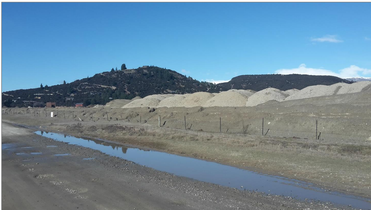
Figure 1: Topsoil stockpiles with no sediment control
