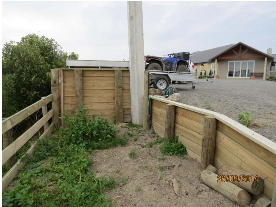
Photo 6: Ground clearance violations in Hastings
