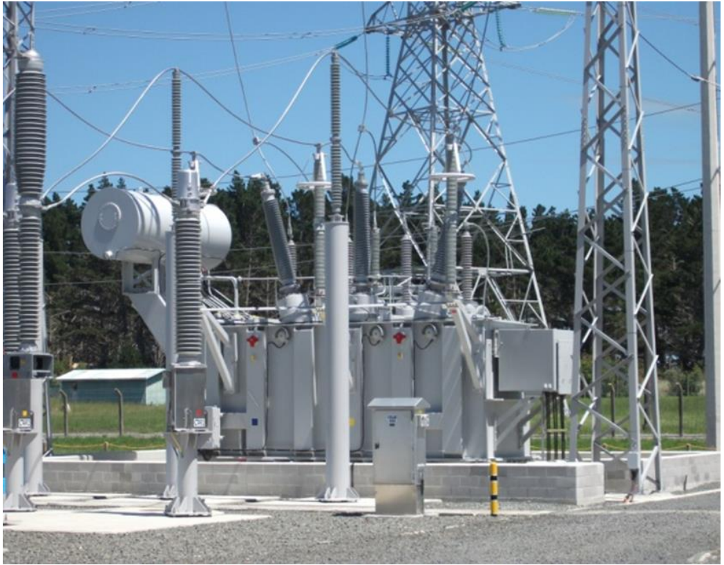
Photo 2: Marsden, Power Transformer
