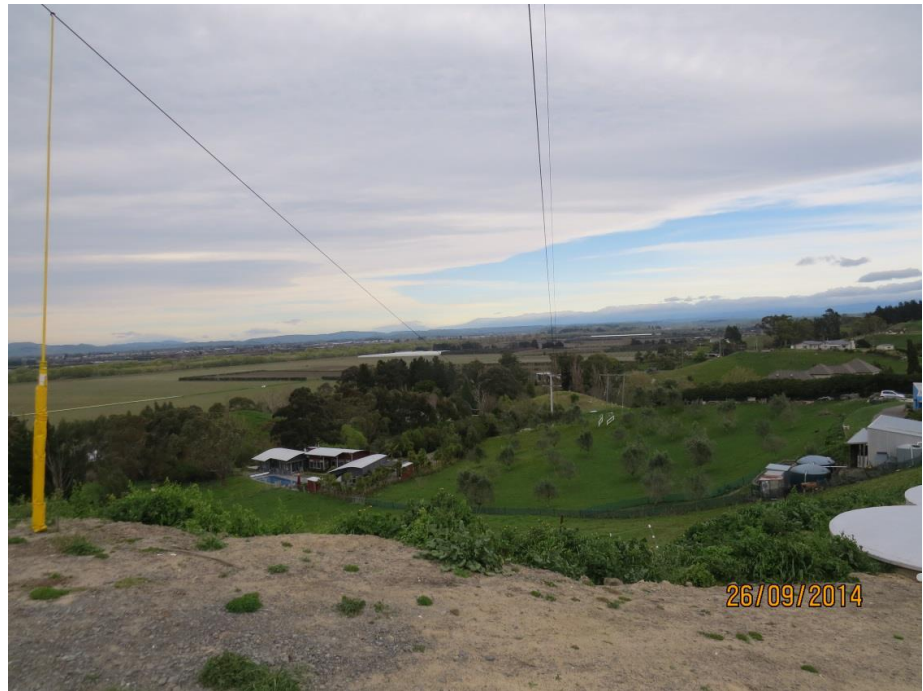
Photo 4: Ground clearance violations in Hastings
