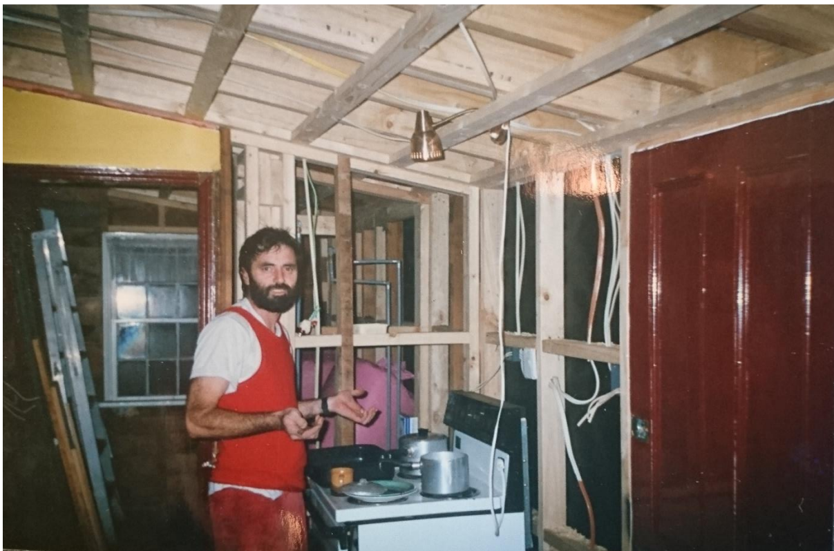
Photo 8 Rebuilding of much of the lean-to and refurbishment c. 1994 – photo supplied by present owners
